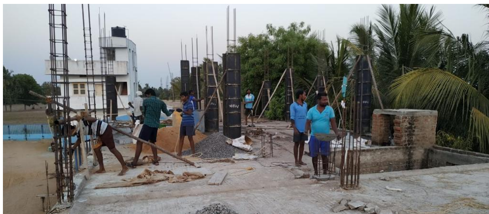
(above) On site during construction of new hall and treatment facilities at Prem Niketan
